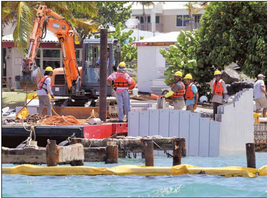
Using a front loader on a barge, construction workers install pilings as work continues on repairs to the main dock at the St. Thomas Yacht Club, which was heavily damaged during Hurricane Irma in September 2017. According to club officials, work on the repairs to
